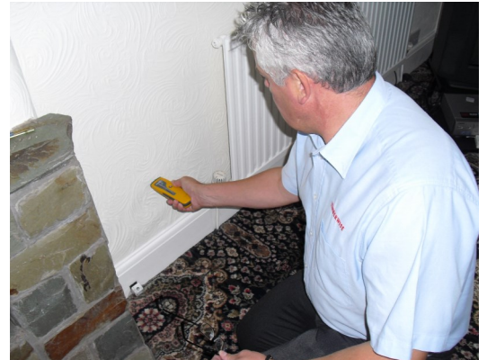
Surveyor Diagnosing For Rising Damp
