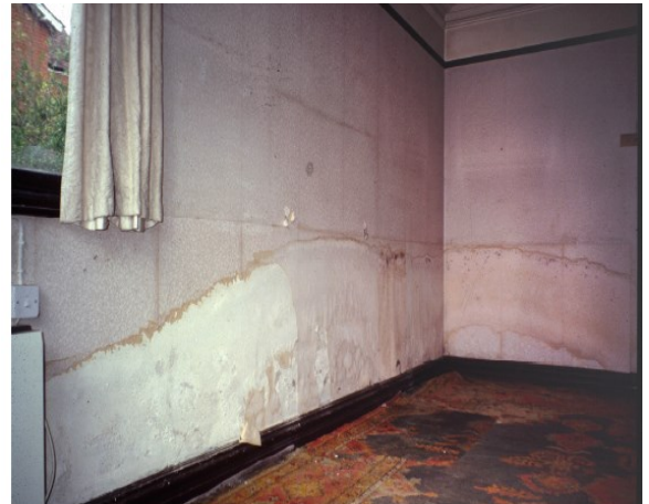
Rising Damp Issue On Interior Wall
