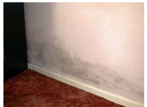
Condensation Mould On Interior Wall
